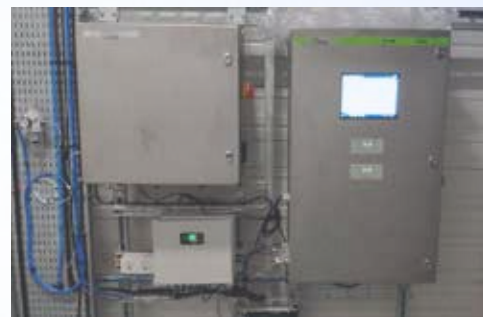
Cabinet for WWTP application
